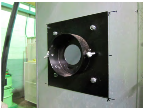
Figure 3. Bracket on gin duct.
