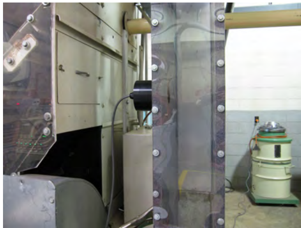
Figure 4. The mass flow sensor installed on a duct behind gin stand.
